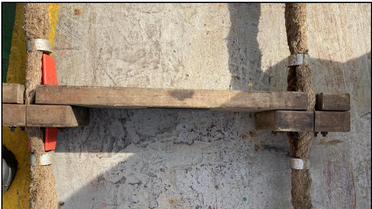
Ladder step replaced and step fixing piece missing.
